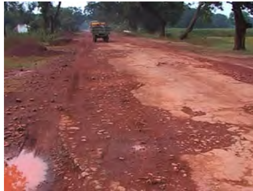
No lane infrastructure
